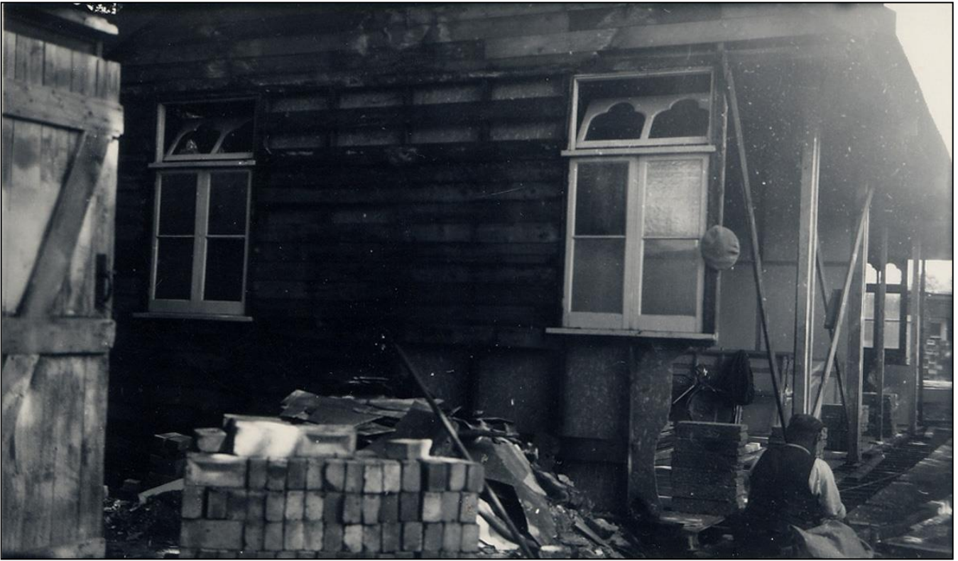
Building the Chapel at Grenham House School – 1954 [Photos taken by A. T. Walker]
